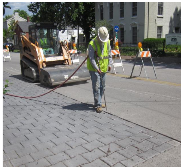
Figure 13. (a) Vacuum maintenance (b) Air jet cleaning method
